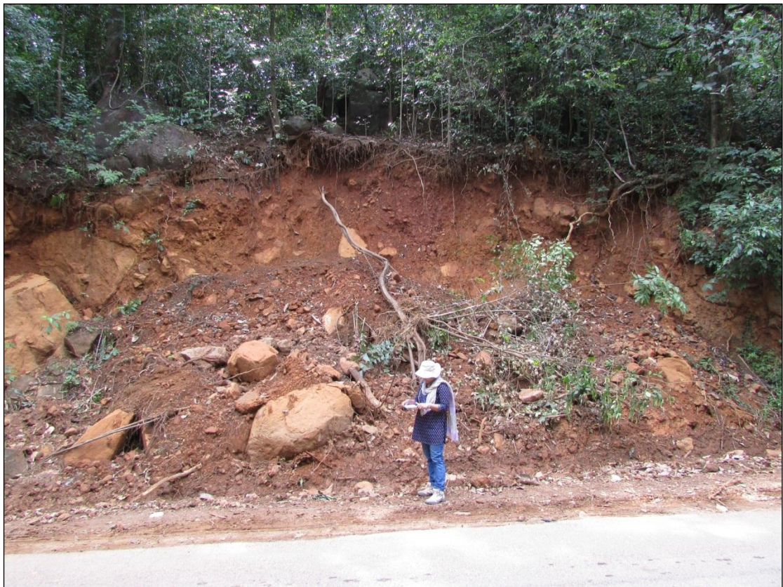
Photo – 4: Active debris slide (Slide Name: KAR/CKM/48O08/2017/053) along Kotighere – Ujire road section in TS no 48O/08 (Latitude - 13^{\circ} 4' 44.61'' N, Longitude - 75^{\circ} 28' 11.12'' E).
