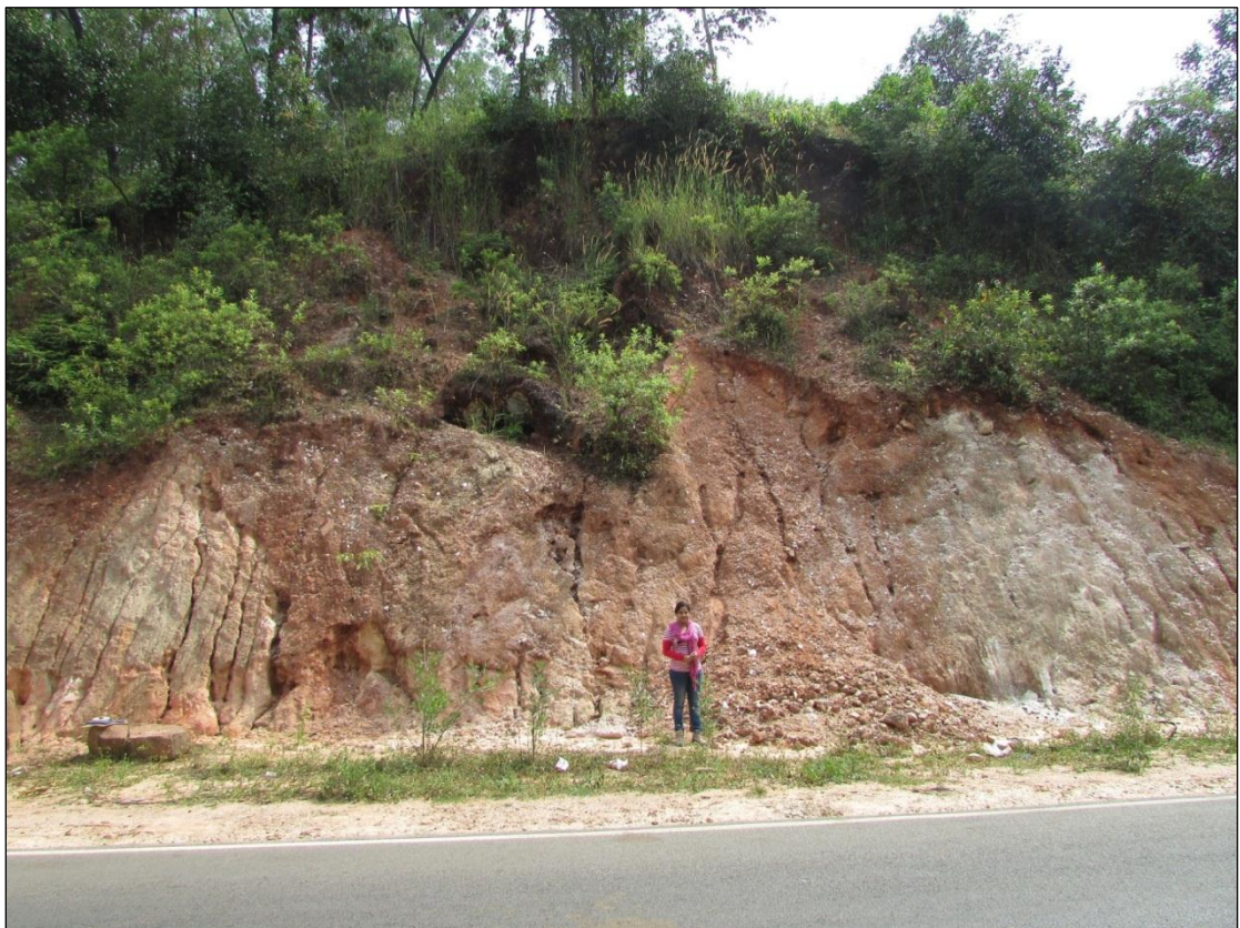
Photo – 6: Extensive Cut Slope near Kalasa along Kalasa – Kotighere road section in TS no 48O/08.
