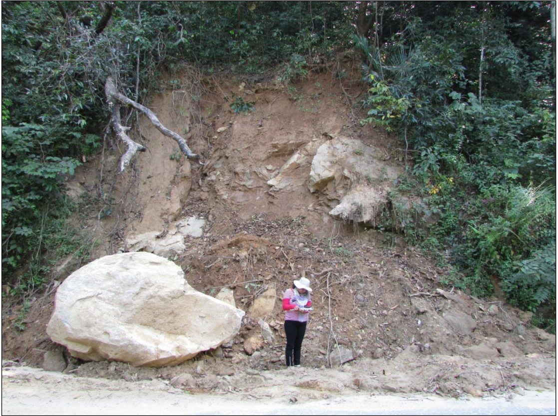
Photo – 5: Active debris slide (Slide Name: KAR/CKM/48O08/2017/077) along Kotighere – Ujire road section in TS no 48O/08 (Latitude - 13^{\circ} 4' 36.88'' N, Longitude - 75^{\circ} 27' 22.63'' E).
